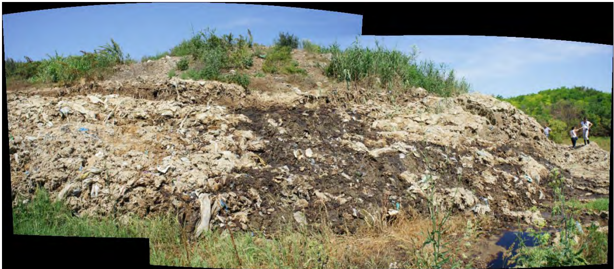
Figure 4.12 - View looking south-east back over the debris flow at the toe of the Vinca Municipal Waste site landslide.
