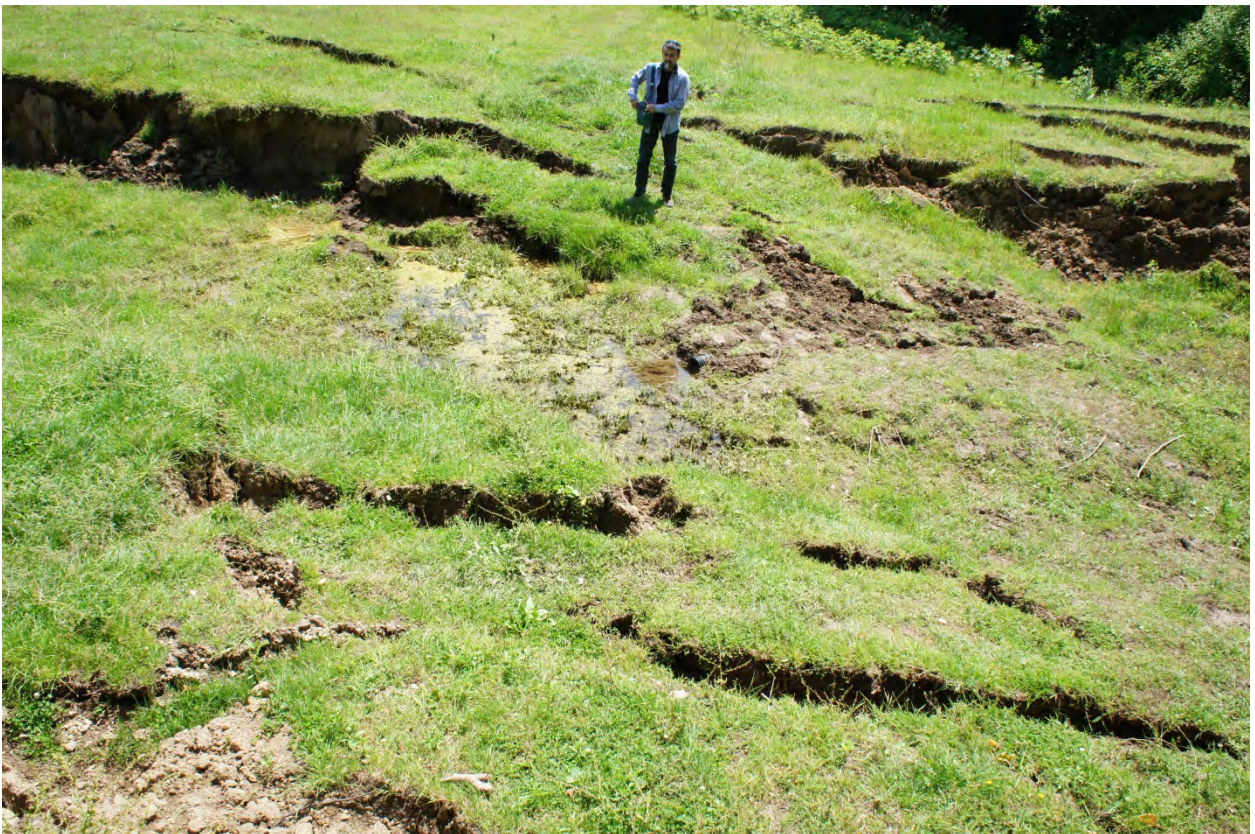
Figure 4.2 - Scarp features seen in the middle of the landslide mass at Mali Zvornik showing the typical features for multiple rotational slides with small pools of water observed.
