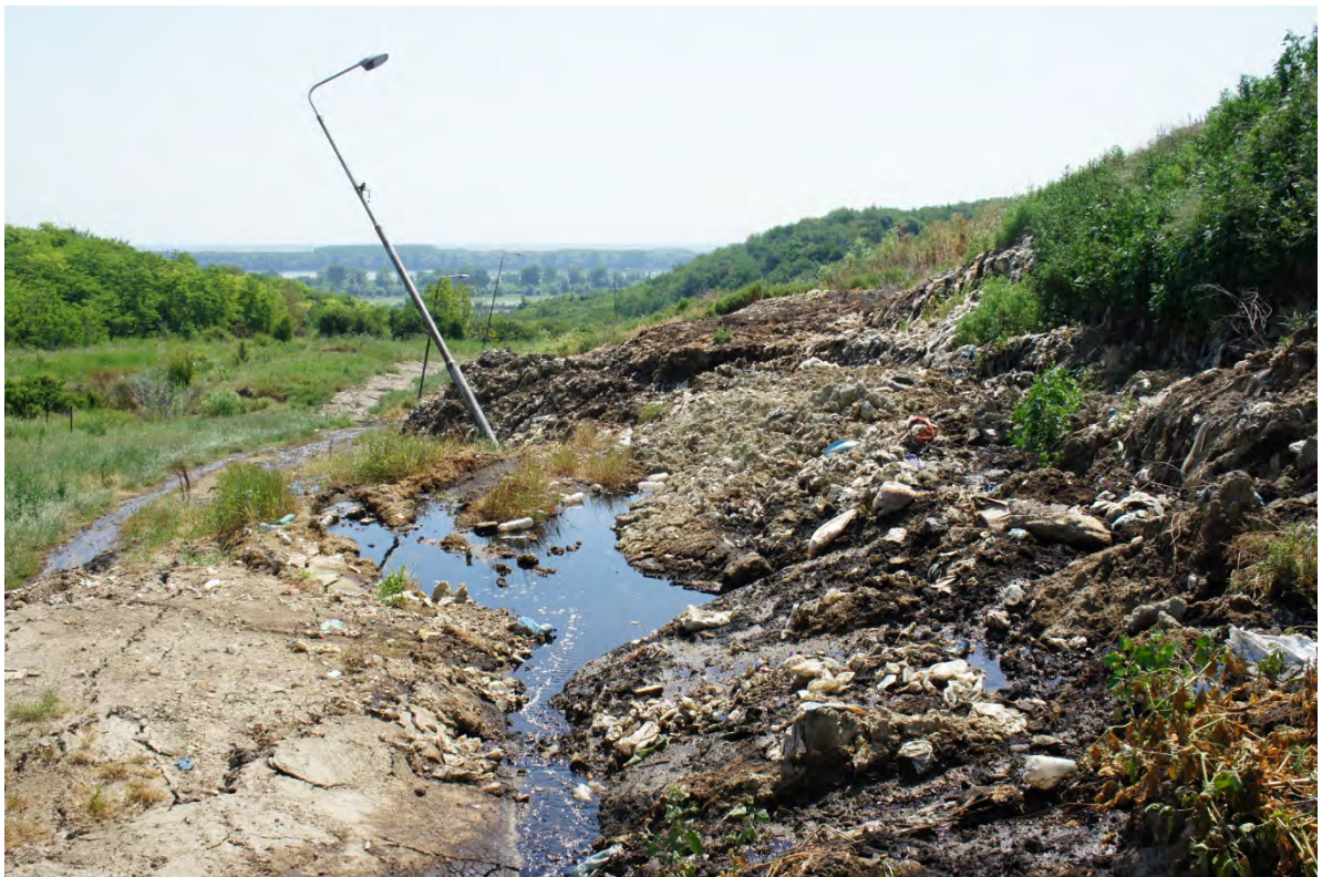
Figure 4.14 - View looking north of the damage to the infrastructure and road around the edge of the Belgrade Municipal Waste Site.
