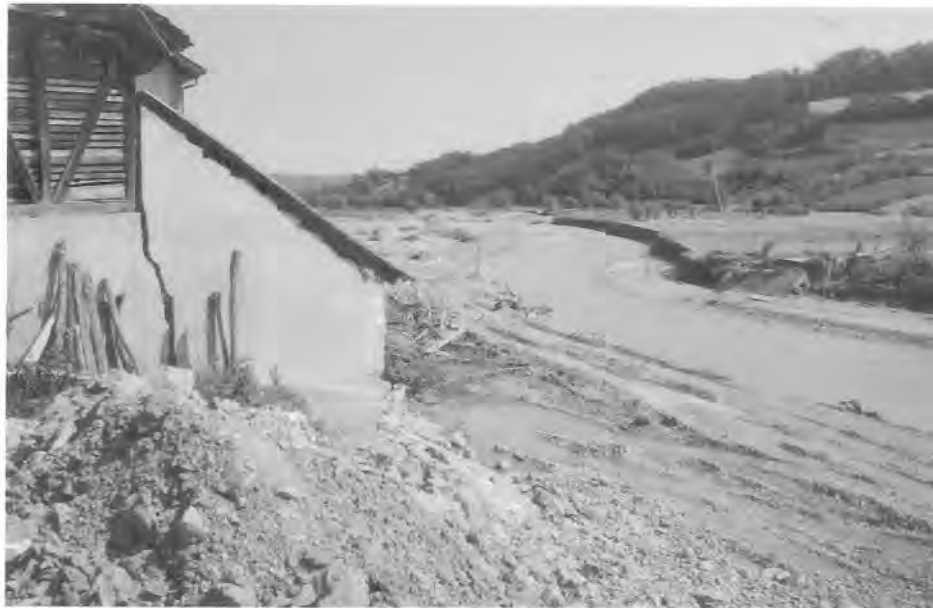
Valley of river Likodra – damaged house in Lipenovic
