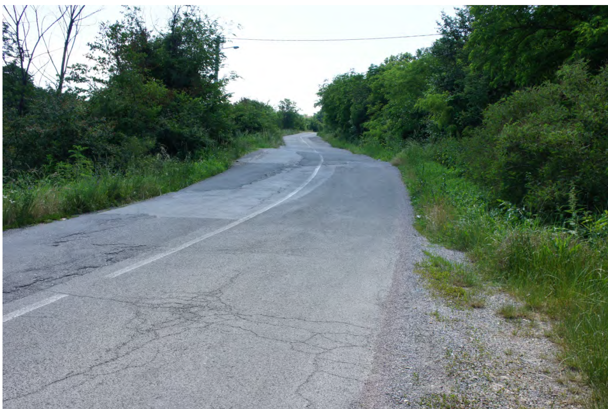
Figure 4.6 - A view of the slow moving rotational landslide observed at Duboko. Damage to road from the slow moving landslide can be observed.
