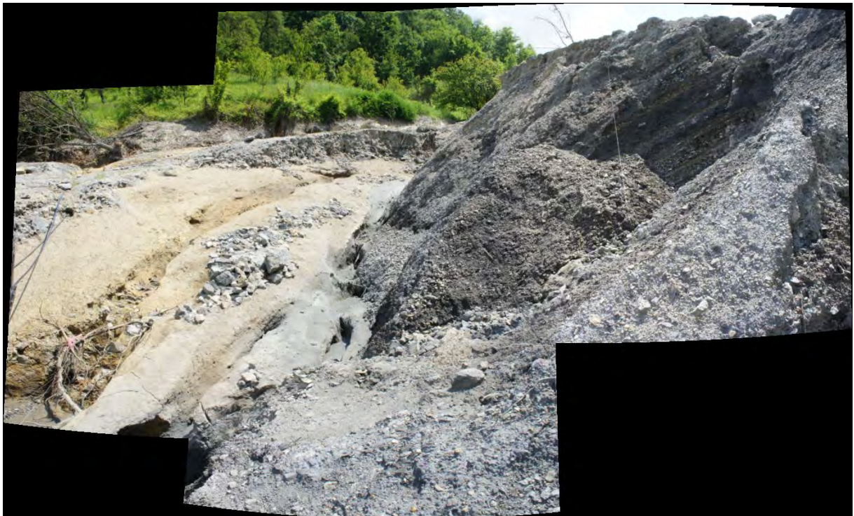
Figure 4.10 - Stolice Antimony Mine Waste Tailings Dam showing breached embankment and discharge of mine waste water.
