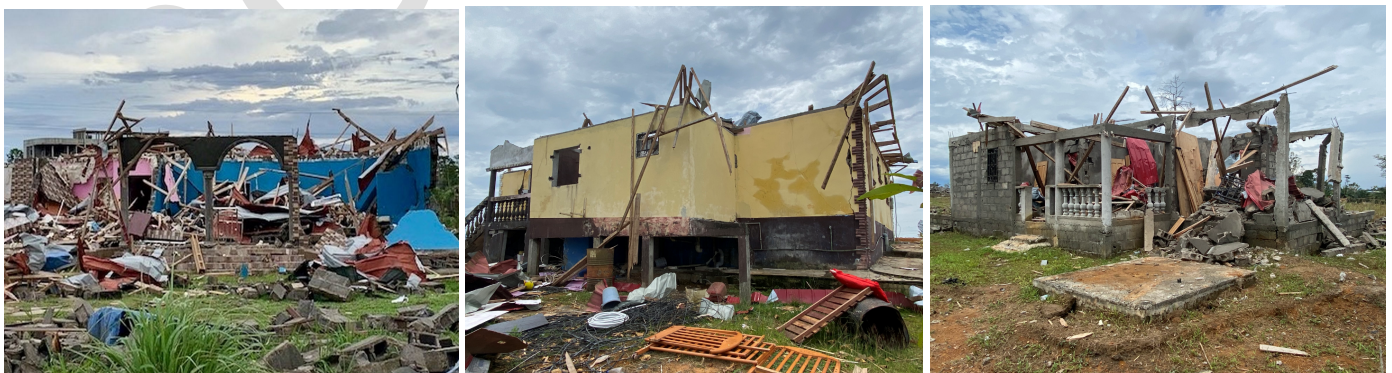
Photo 15 -17: Buildings affected by the explosions in Bata
